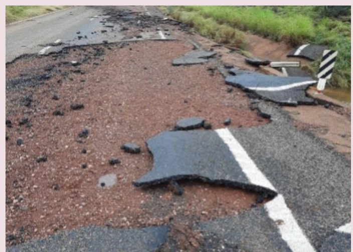
Landsborough Highway (Kynuna–Cloncurry) – seal delamination at floodway
