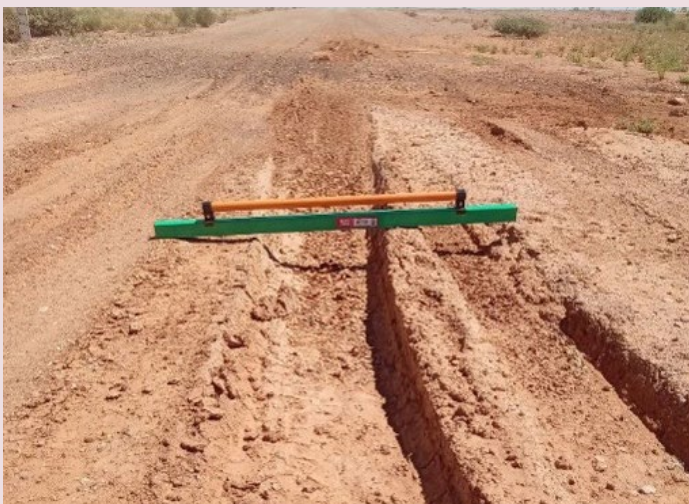
Diamantina Developmental Road (Windorah–Bedourie) – severe rutting
