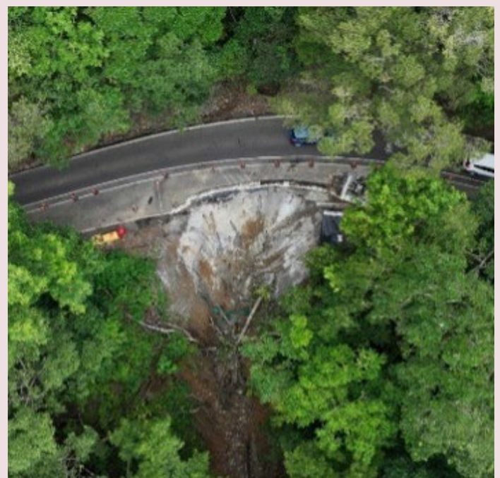
Kuranda Range Road – landslip site (March 2024).
