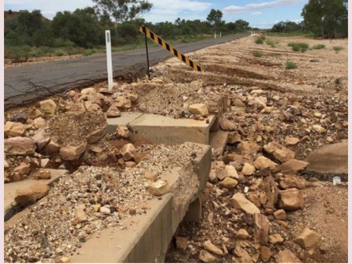
Kennedy Developmental Road (Winton–Boulia) – culvert damage
