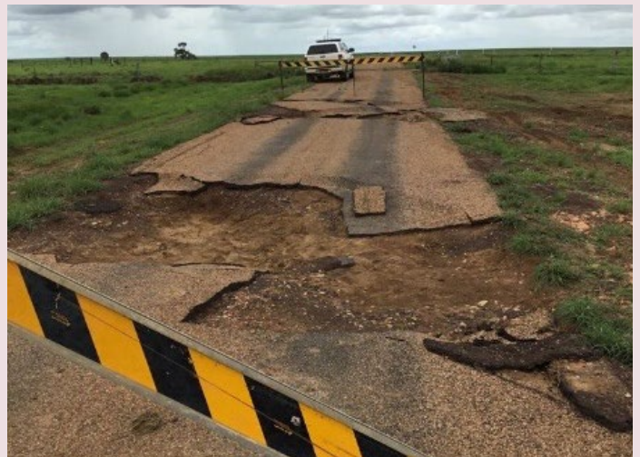
Kennedy Developmental Road (Winton–Boulia) – pavement damage
