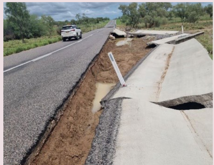
Landsborough Highway (Kynuna–Cloncurry) – concrete batter damage at Wild Duck Creek
