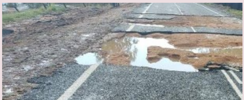
Booyal–Dallarnil Road – pavement damage caused by South East Queensland Rainfall and Flooding (February 2022)
