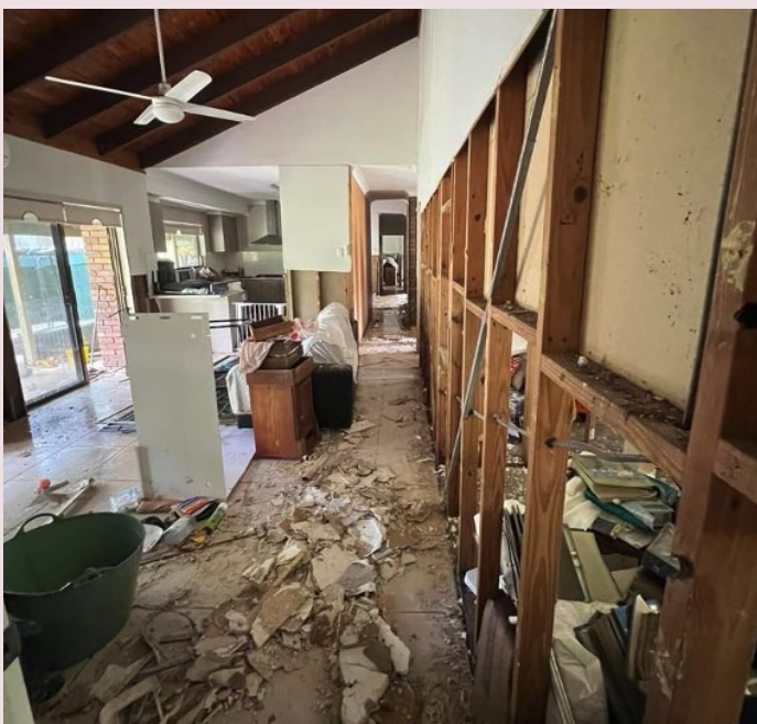
Aftermath of the floods, Keith Roxburgh’s Morayfield home was severely damaged.
