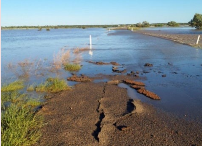
Wills Developmental Road – pavement damage due to long-term inundation
