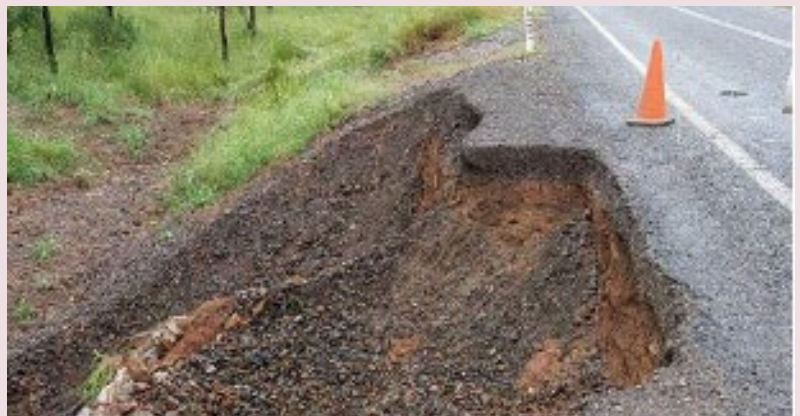
Booyal–Dallarnil Road – culvert damage caused by South East Queensland Rainfall and Flooding (February 2022)
