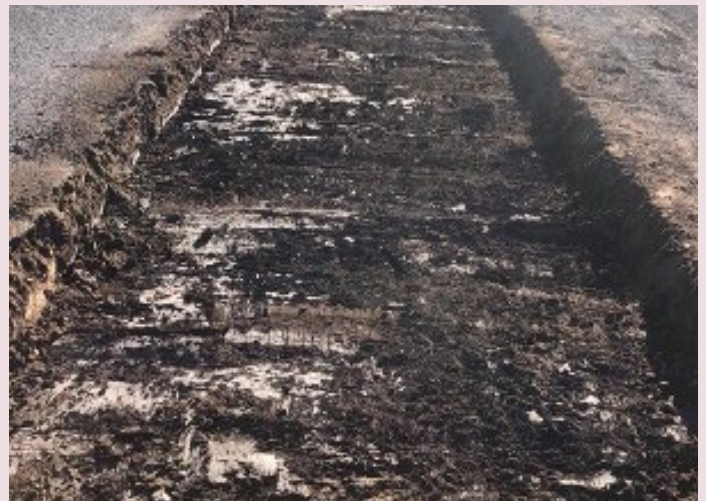
Toowoomba–Cecil Plains Road – black soil subgrade at Evanslea Floodway
