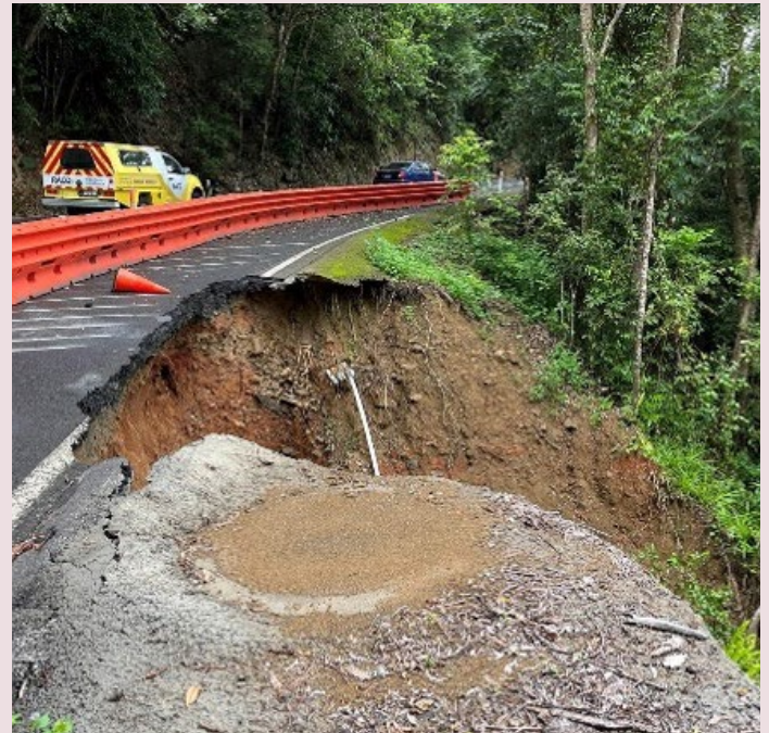
Kuranda Range Road – landslip site (February 2024).
