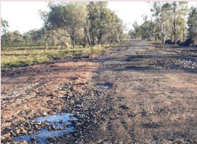
Toowoomba–Cecil Plains Road – pavement delamination from Southern Queensland Flooding event (May 2022)
