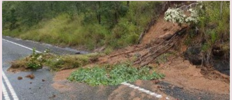
Booyal–Dallarnil Road – batter slip caused by Ex-Tropical Cyclone Seth (January 2022)
