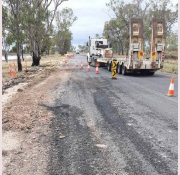
Toowoomba–Cecil Plains Road – pavement damage near Condamine River from Central, Southern and Western Queensland Rainfall and Flooding (December 2021)
