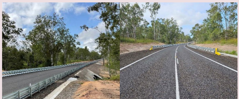
Booyal–Dallarnil Road – completed works at Stoney Creek prior to line marking (April 2024)
