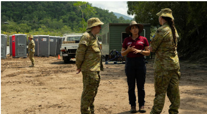
Inspecting the progress of resupply and restoration of the Ayton Boat Ramp, Ayton, Cook Shire
