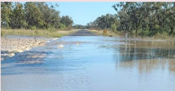
Castlereagh Highway (St George–Hebel) – water over road following Southern Queensland Flooding event (May 2022)
