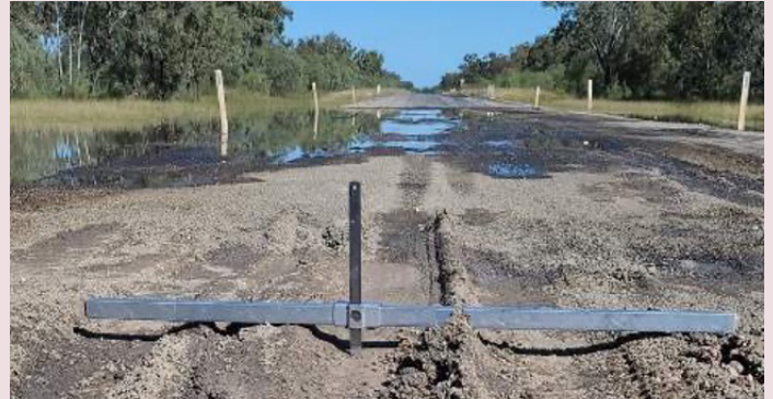
Castlereagh Highway (St George–Hebel) – pavement damage (May 2022)
