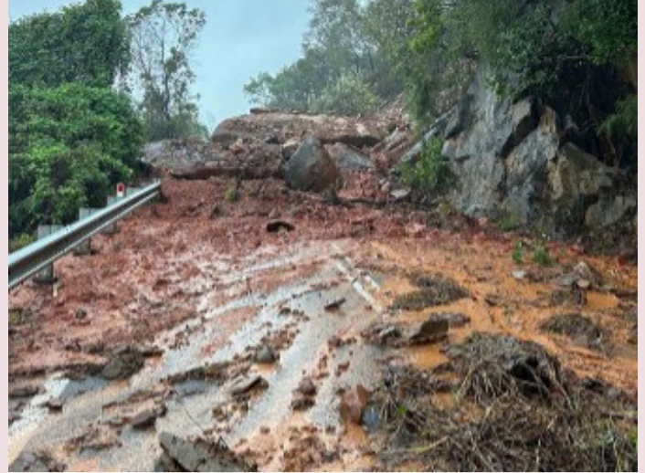
Captain Cook Highway (Cairns–Mossman) – landslip at Buchans North caused by Tropical Cyclone Jasper (December 2023)
