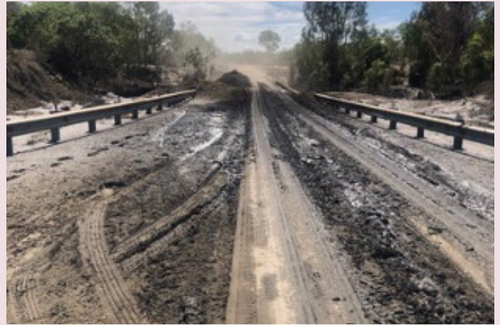
Mulligan Highway – silt build-up caused by TC Jasper (December 2023)
