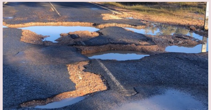
Castlereagh Highway (St George–Hebel) – pavement damage at floodway (June 2022)
