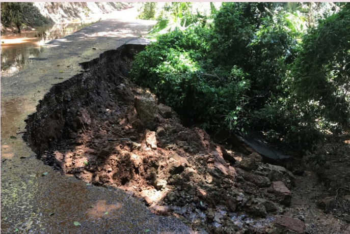
Shiptons Flat Road – damage caused by TC Jasper (December 2023)
