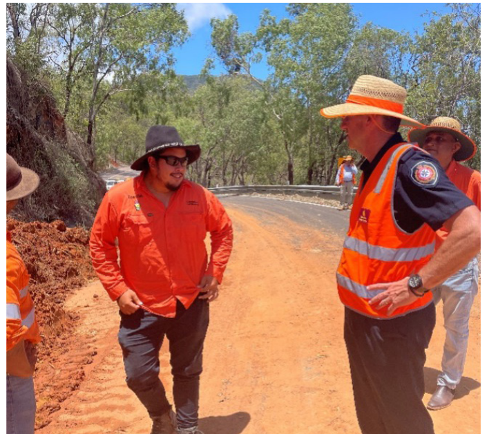
Deputy State Recovery Coordinator, Deputy Commissioner Mike Wassing receiving a briefing from Department of Transport and Main Roads crews working to re-open the Captain Cook Highway
