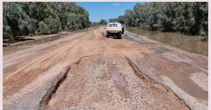
Castlereagh Highway (St George–Hebel) – pavement damage at floodway (November 2022)
