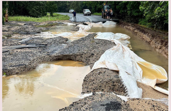
Mossman–Mount Molloy Road – damage from TC Jasper (December 2023)
