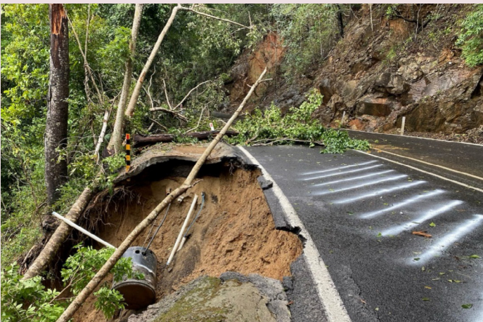
Kuranda Range Road – landslide and exposed ITS equipment following TC Jasper (December 2023)
