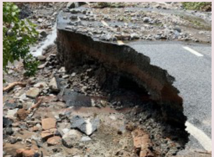
Captain Cook Highway (Cairns–Mossman) – major pavement damage caused by TC Jasper (December 2023)
