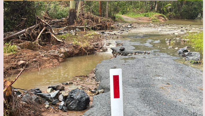
The south-east also suffered washouts from the floods.
