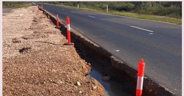
Castlereagh Highway (St George–Hebel) – shoulder scouring at floodway (May 2022)
