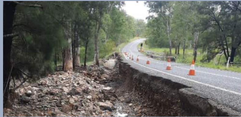
Image: Isis Highway (Childers–Biggenden) – severe shoulder scouring caused by SEQ Rainfall and Flooding.
