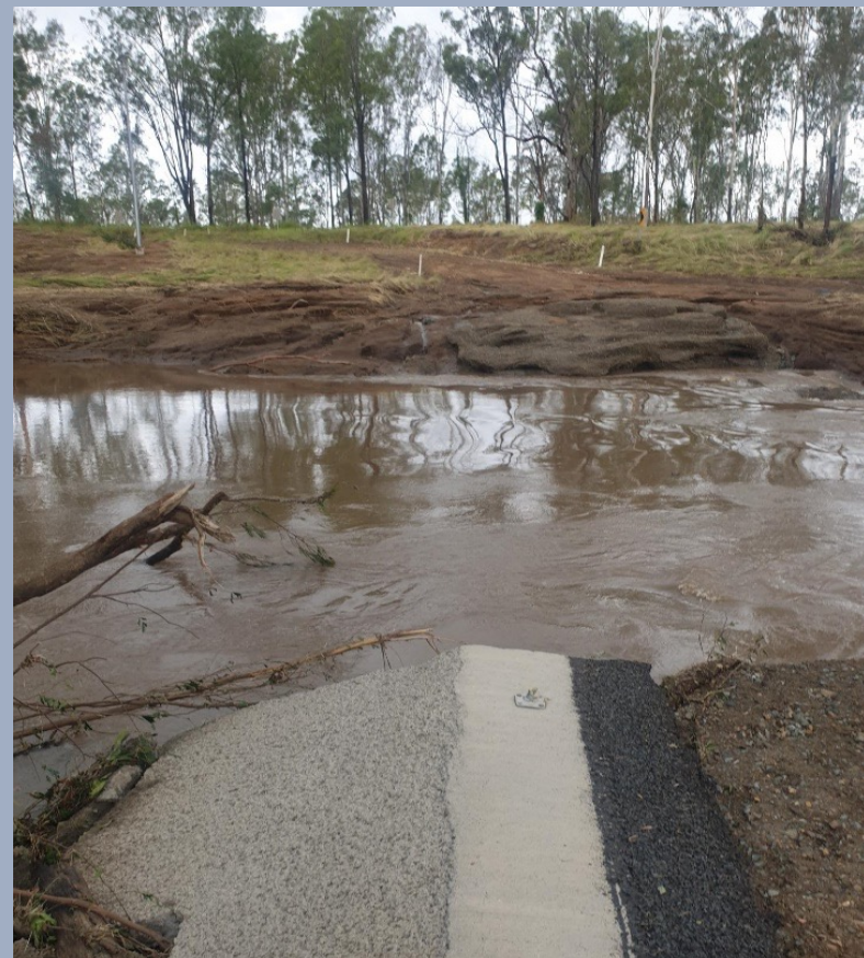
Image: Brooweena–Woolooga Road – damage at Running Creek following ex-TC Seth (January 2022).
