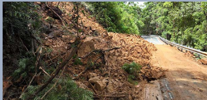
Image: Gold Coast–Springbrook Road – landslide caused by SEQ Rainfall and Flooding.
