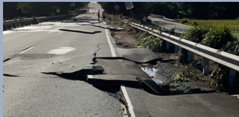
Image: Brisbane–Woodford Road at Bald Hills Flats – pavement damage from SEQ Rainfall and Flooding.
