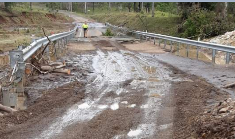
Image: Brooweena–Woolooga Road – damage at Spring Creek following ex-TC Seth (January 2022).
