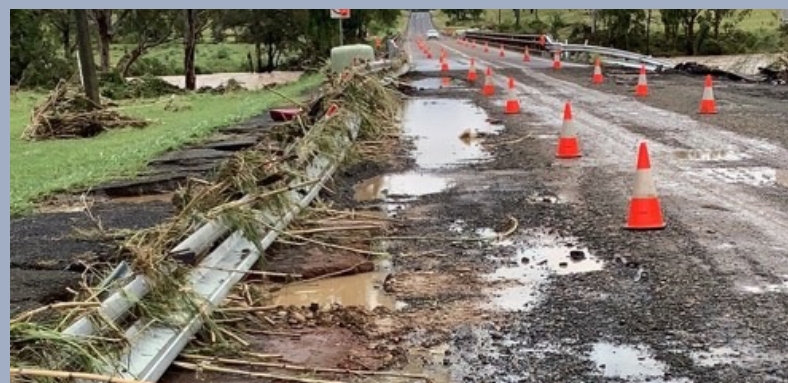
Image: Gatton–Clifton Road – damage from SEQ Rainfall and Flooding.
