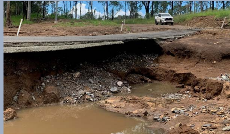
Image: Brooweena–Woolooga Road – damage at Running Creek caused by the SEQ Heavy Rainfall and Flooding event (February 2022).
