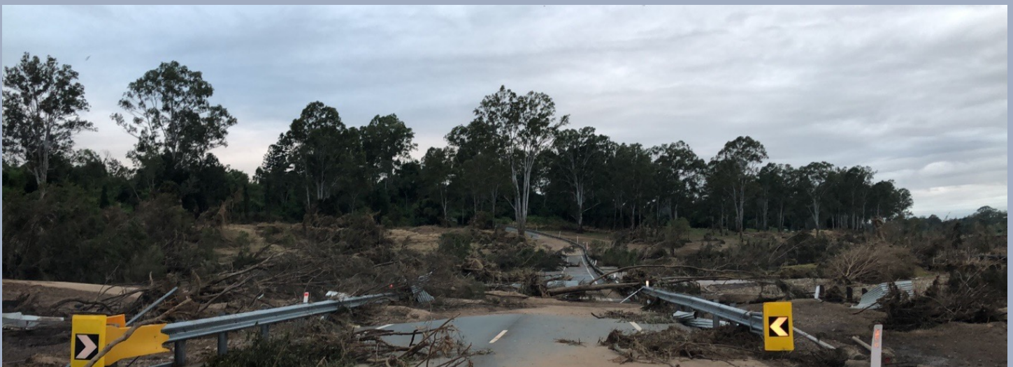
Image: Colleges Crossing after the water receded.
