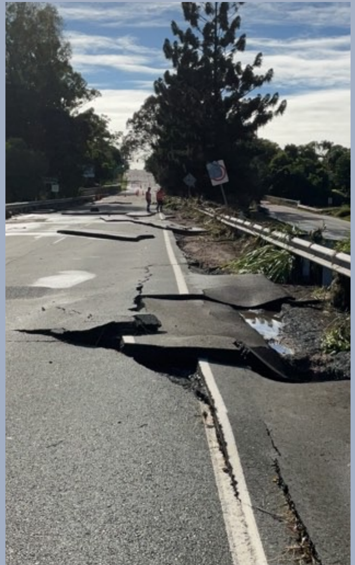
Photo: Brisbane–Woodford Road at Bald Hills Flats – damage from SEQ Rainfall and Flooding.
