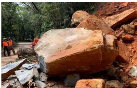
Mount Spec Road – large boulders had to be broken down and removed from the road
