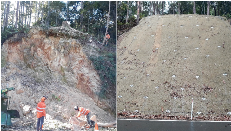
Photos Above: Tomewin Mountain Road – site 8969 damage and completed work
