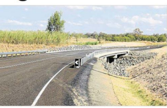
SOLID AS A ROCK: The Thistlethwaite Bridge at Grantham reopened to traffic last Friday.
