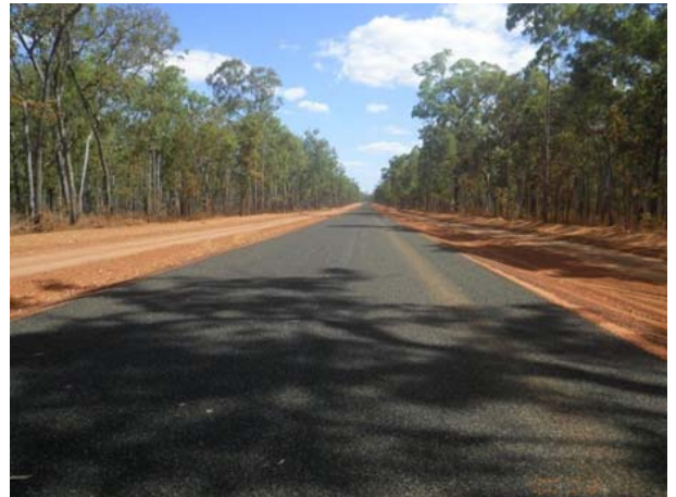
Damage to Aurukun Access Road (top); and on completion (bottom) of reconstruction and betterment works (bottom)
