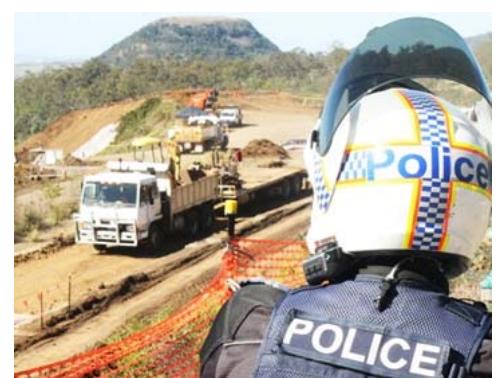
Large load approaching a Darling Downs worksite (top) and police patrol on Toowoomba Range (bottom)
