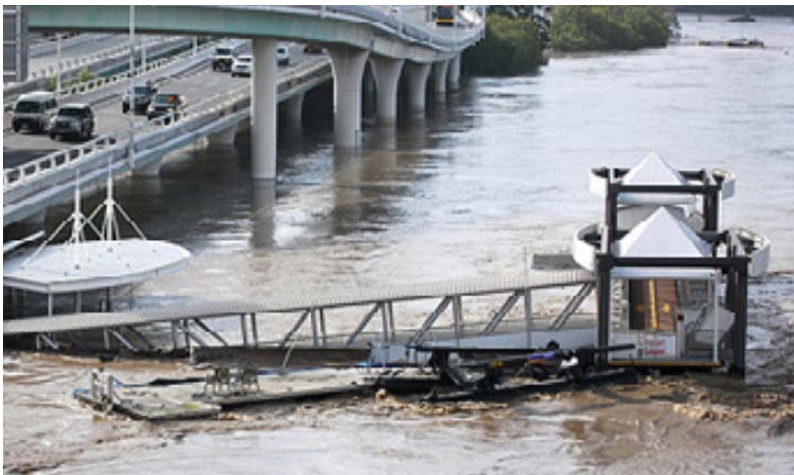
Damage to the North Quay terminal during the 2011 flood event
