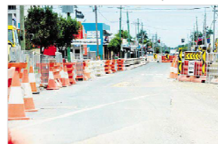
NEW WORK: The last of the Natural Disaster Relief and Recovery Arrangements funded roadworks have to be completed by June 30. PHOTO: TONY MARTIN
