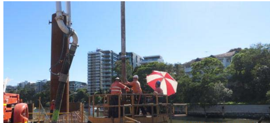
Concrete being poured into one of the piles that are embedded into the riverbed
