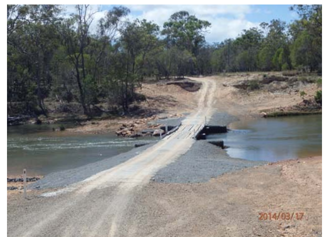
Top: damage to Worthington Creek bridge following 2011 flood event —April 2011
