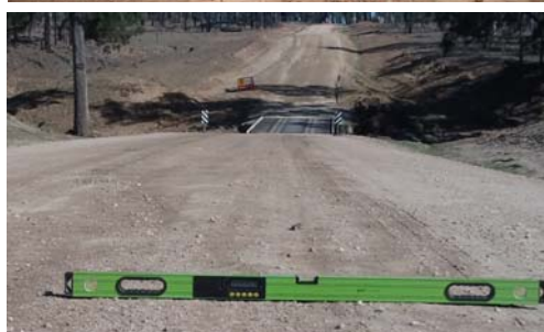
Damage (top and centre) and nearing completion of works (bottom) to Gregory Springs Road
