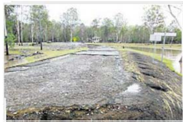
TORN UP: Widgee road damage following last year's flooding.
