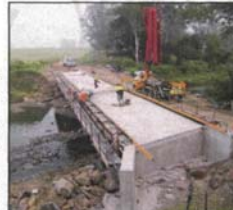
Construction on a new concrete bridge on Foggs Road at Harlin is almost complete.
