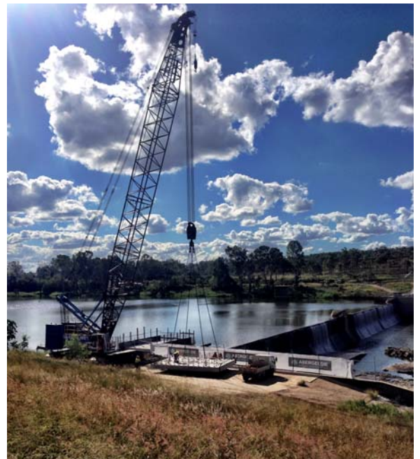
Right: Stage two works underway at Claude Wharton Weir to Gayndah Water Supply Intake Station betterment project - May 2014
