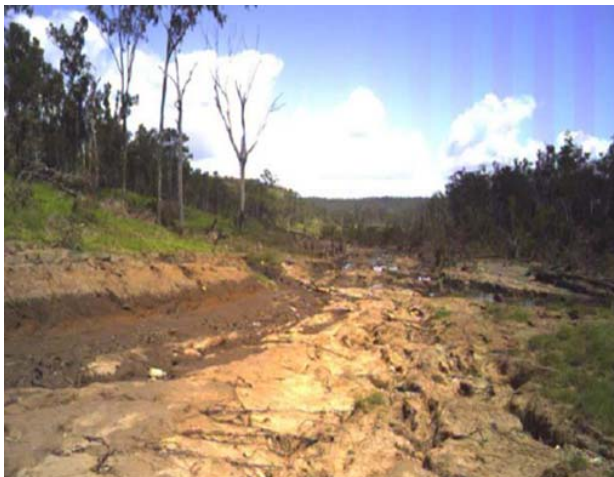
Above: damage to the Gayndah-Mundubbera Road following flooding associated with Tropical Cyclone Oswald in early 2013
