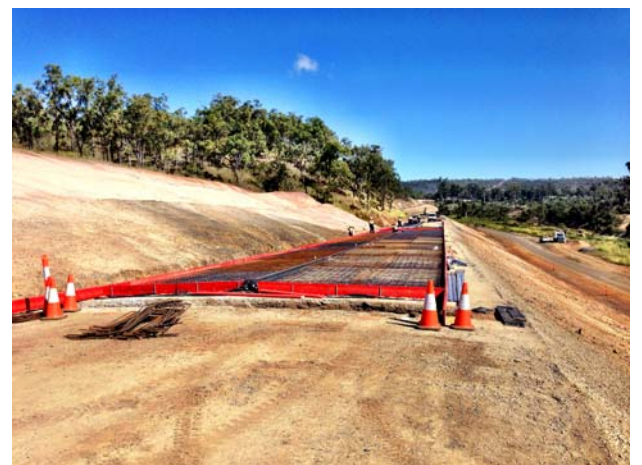
Right: Construction works underway to the Gayndah - Mundubbera Road betterment project - May 2014
