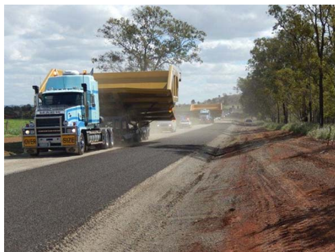
Above: Isis Highway (Biggenden to Coalstoun Lakes) – wide loads traversing partially sealed site
