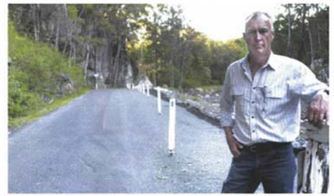
Cr Rick Stanfield stands on a reconstructed section of The Head Road at Carney's Creek where flood waters undermined the road surface. The road up to Teviot Falls and on to Killamey is now open.
