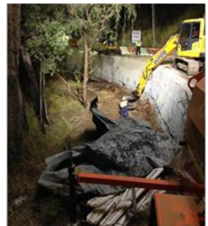
Night works to install soil nails near a one-way section of the road
