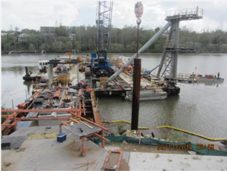
Gangway portal and marine works underway at University of Queensland ferry terminal
