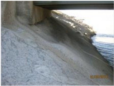
Damage to (top) and following reconstruction works (bottom) on Heatleys Parade bridge which was repaired using Townsville City Council's day labour workforce.
