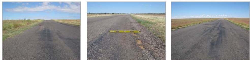
Above: showing damage to sections of Cannington Road.
