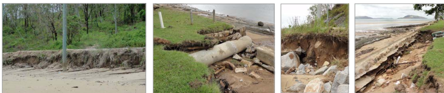
Images above showing damage to sections of Palm Island the seawall following Tropical Cyclone Yasi.
