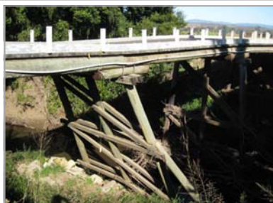
Right: showing damage to the old timber Stokes Bridge.
