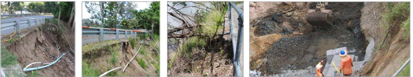
Images above: showing damage at the creek bank and progress of reconstruction works to infrastructure supporting Radnor Street.
