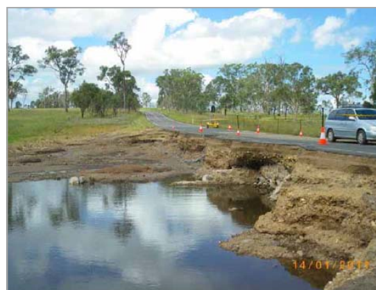
Above: Damaged section of the Burnett Highway (Nanango - Goomeri) at Barambah Creek (Image courtesy TMR)
