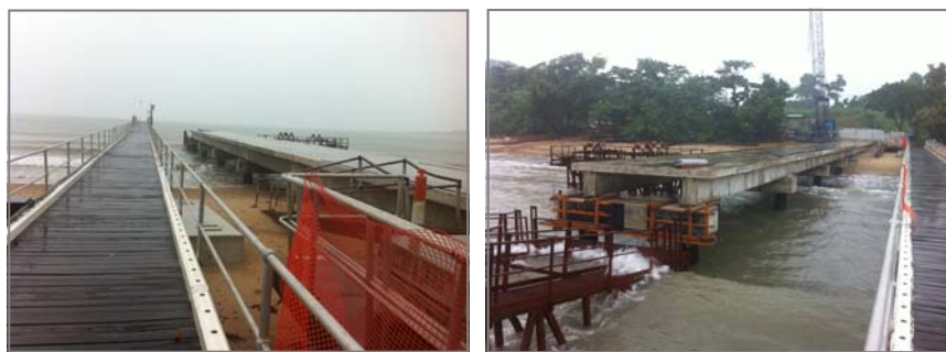
Above: Recent photos showing progress of works on the new Clump Point jetty
