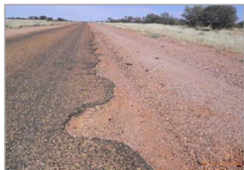
Above: damage to a section of Diamantina Development Road.
