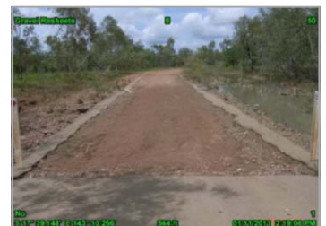
Above: damage to sections of the road to Abingdon Downs.
