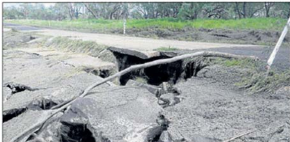
TORN UP: Magenta Langton Road was one of 2500 sites to be repaired over the next nine months after damage in 2015 storms. Picture: Central Highlands Regional Council.
