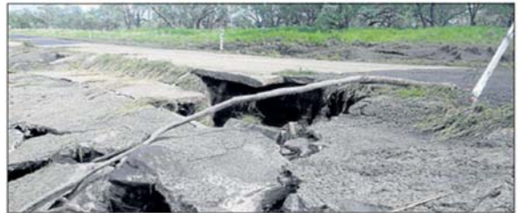
TORN UP: Magenta Langton Road was one of 2500 sites to be repaired over the next nine months after damage in 2015 storms. Picture: Central Highlands Regional Council.
