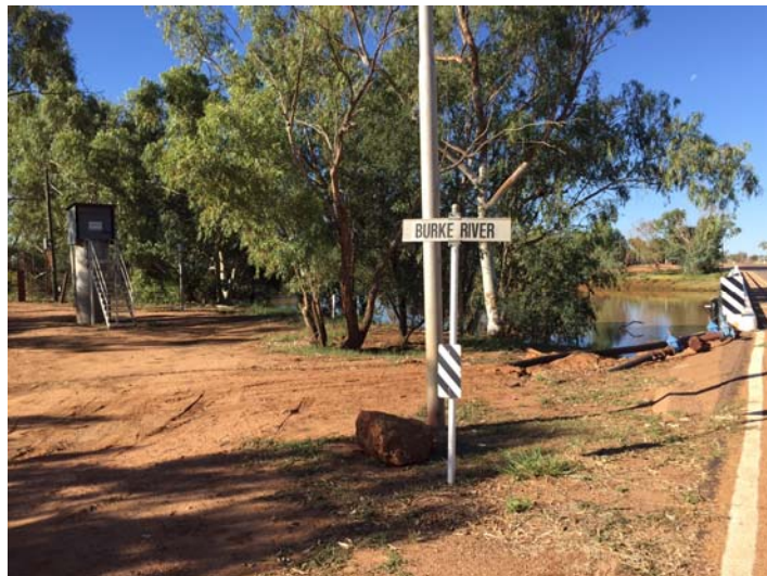
Burke River flood warning gauge at Boullia
