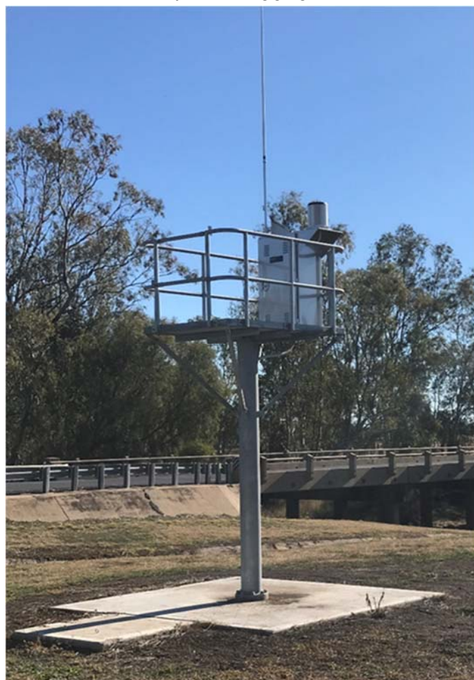
Flood warning gauge in Warra, Western Downs Regional Council
