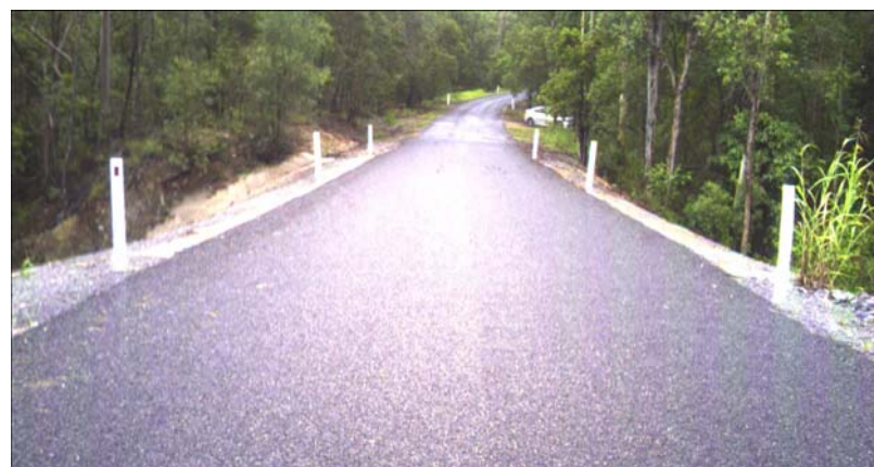
Damage to Monduran Dam Access Road following excessive velocity of floodwater (top) and after the completion of Betterment works making the road more disaster resilient.
