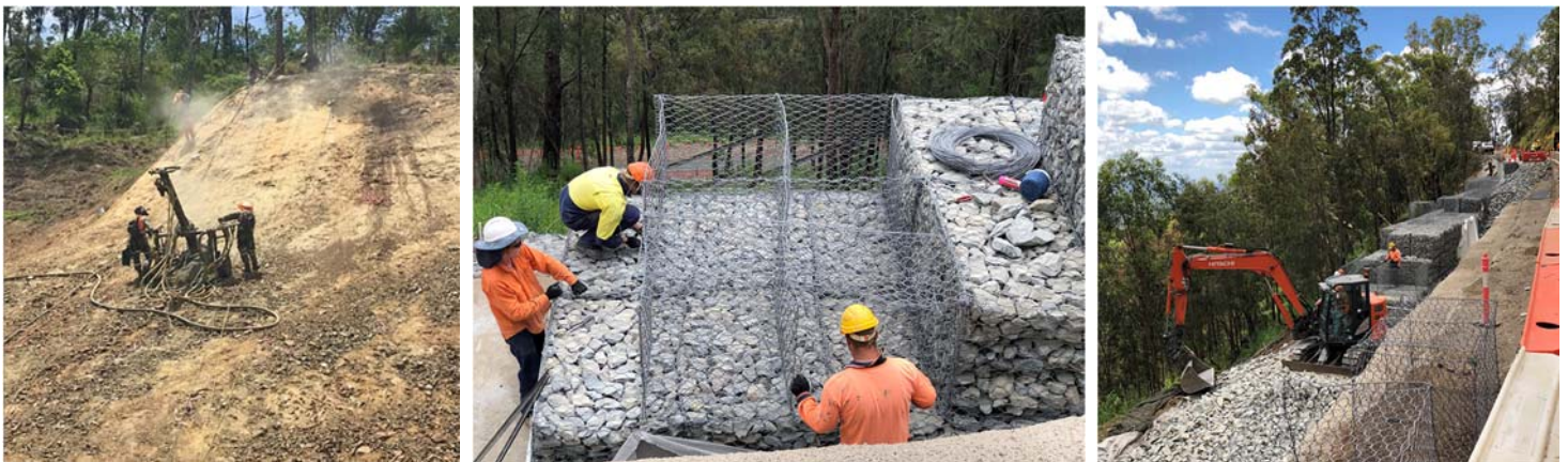
Disaster reconstruction works underway by TMR during December 2017 following impacts of STC Debbie: Soil nailing on upper slope on the Sarina Range (left); installing gabion baskets Lamington National Park Road (middle & right)
