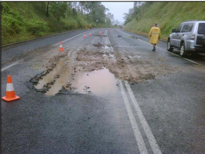
Above: Bruce Highway north of Bloomsbury at Gibson Creek during the 2010/11 wet weather event
